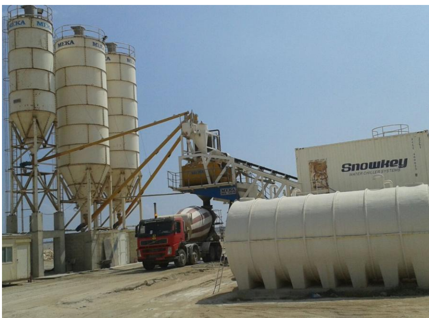
MEKA Mobile Plant : Erected in 2013 Capacity 120m 3 /hr.
