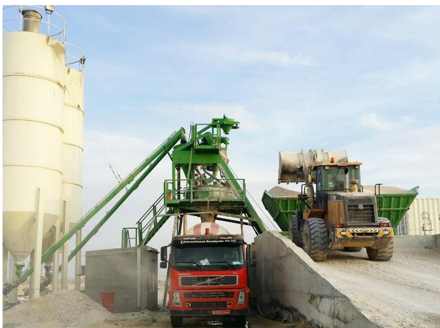
STETTER Semi Mobile Plant : Erected in 2013 Capacity 56m 3 /hr.
