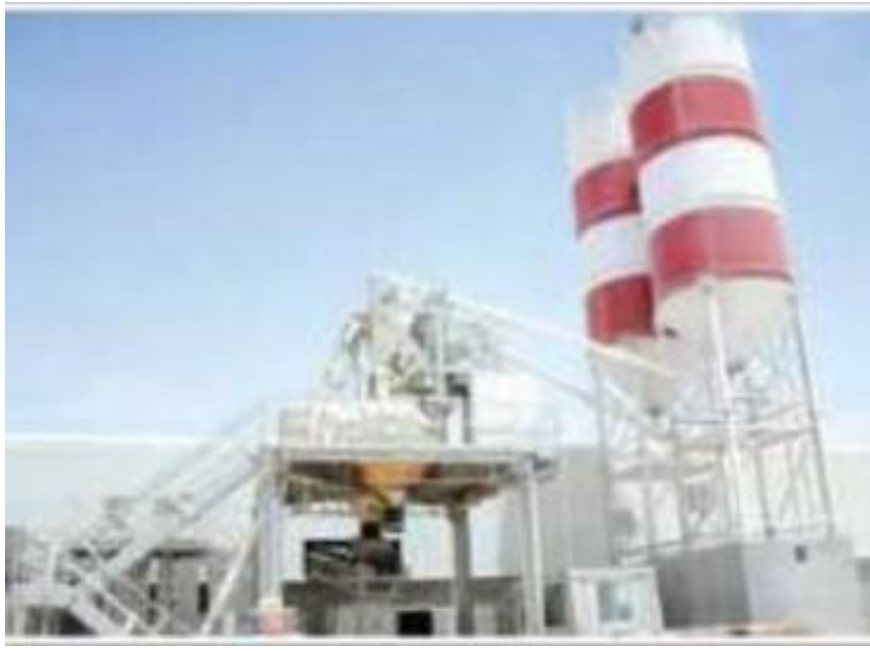
SIMEM Stationary Plant : Erected in 2012 Capacity 60m 3 /hr
